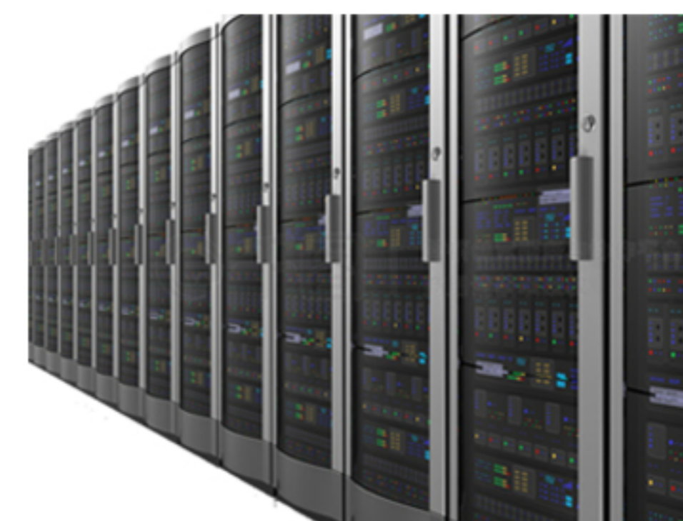
■ Server Power Supply
